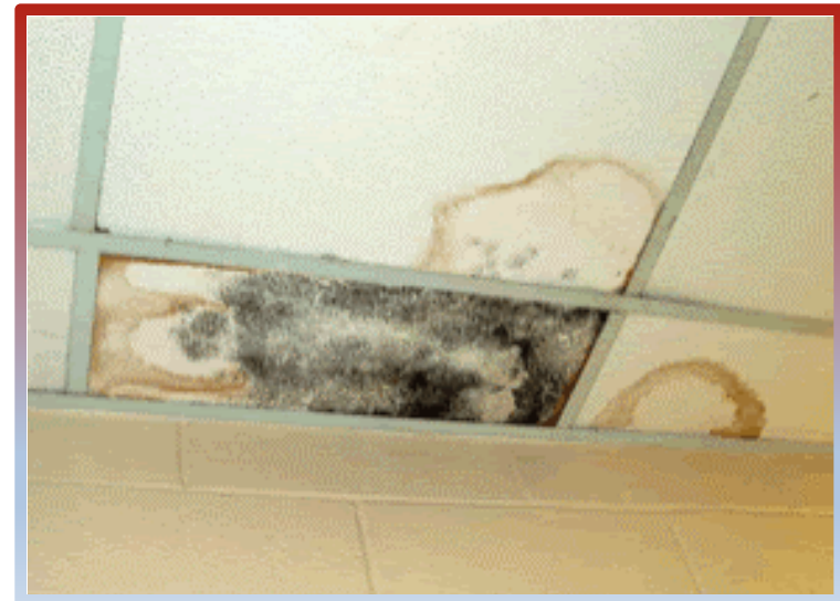
Mould on ceilings
